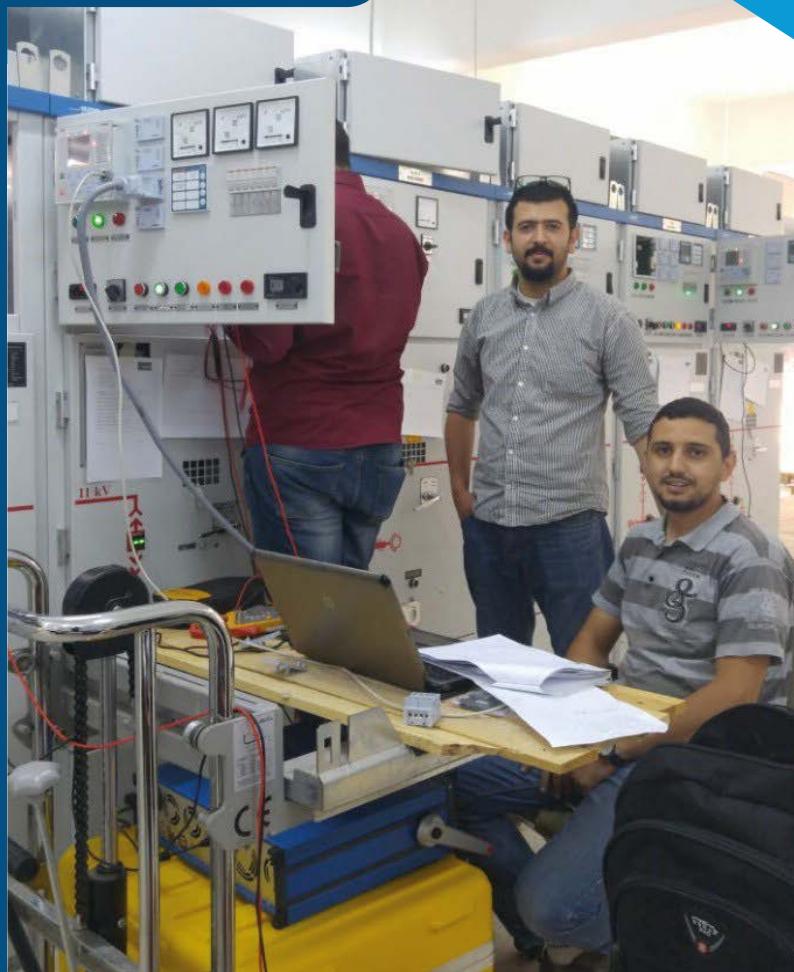
EDCO 33KV Substation
